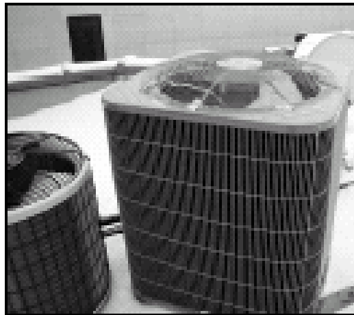
Air conditioning systems
