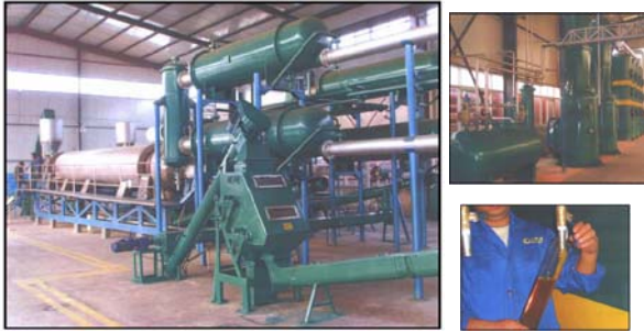
Figure 8. Pyrolysis Plant (Plastic waste to Oil)
